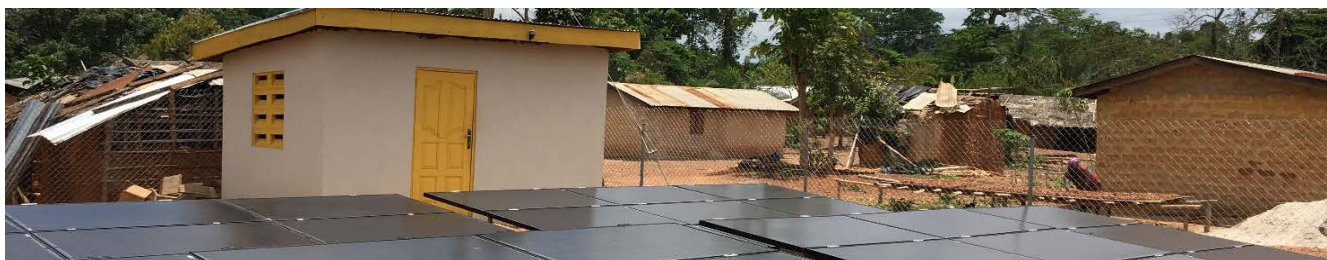
Mini-grids, like this one built by Black Star Energy Ltd., are providing affordable, sustainable electricity to rural Ghanaians for the first time. (Photo: PATRP)
