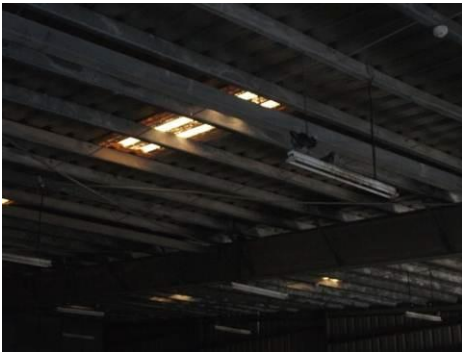
Photo no. 20: Birds Roosting on a Light Fixture Warehouse in the Free Zone in Djibouti
