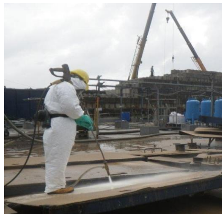
Cleaning equipment in the liquid vapor treatment plant. (Photo: CDM Smith)
