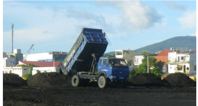
Placing treated soil/sediment into stockpiles for future use by the Vietnamese Ministry of National Defense. (Photo: CDM Smith)
