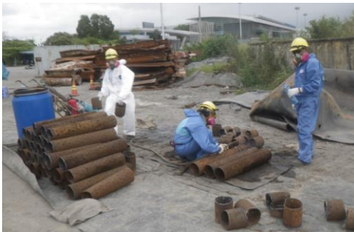
Cleaning leachate pipes that were removed from the bottom of the treatment pile structure. (Photo: CDM Smith)
