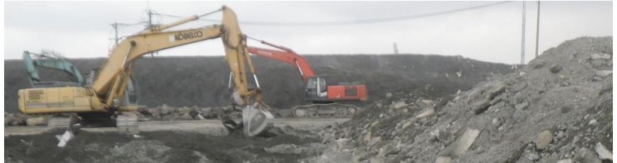
Removing bottom layers of the treatment pile structure for disposal. (Photo: CDM Smith)
