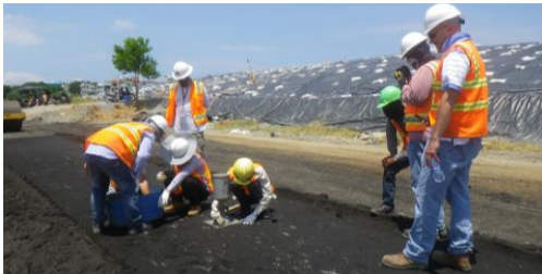
Mixing, compacting, and testing geotechnical properties of treated soil and light weight concrete. (Photo: CDM Smith)
