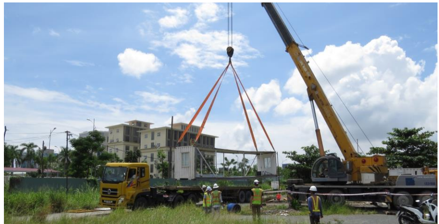
Loading site office trailers onto trucks for removal from the project site. (Photo: CDM Smith)
