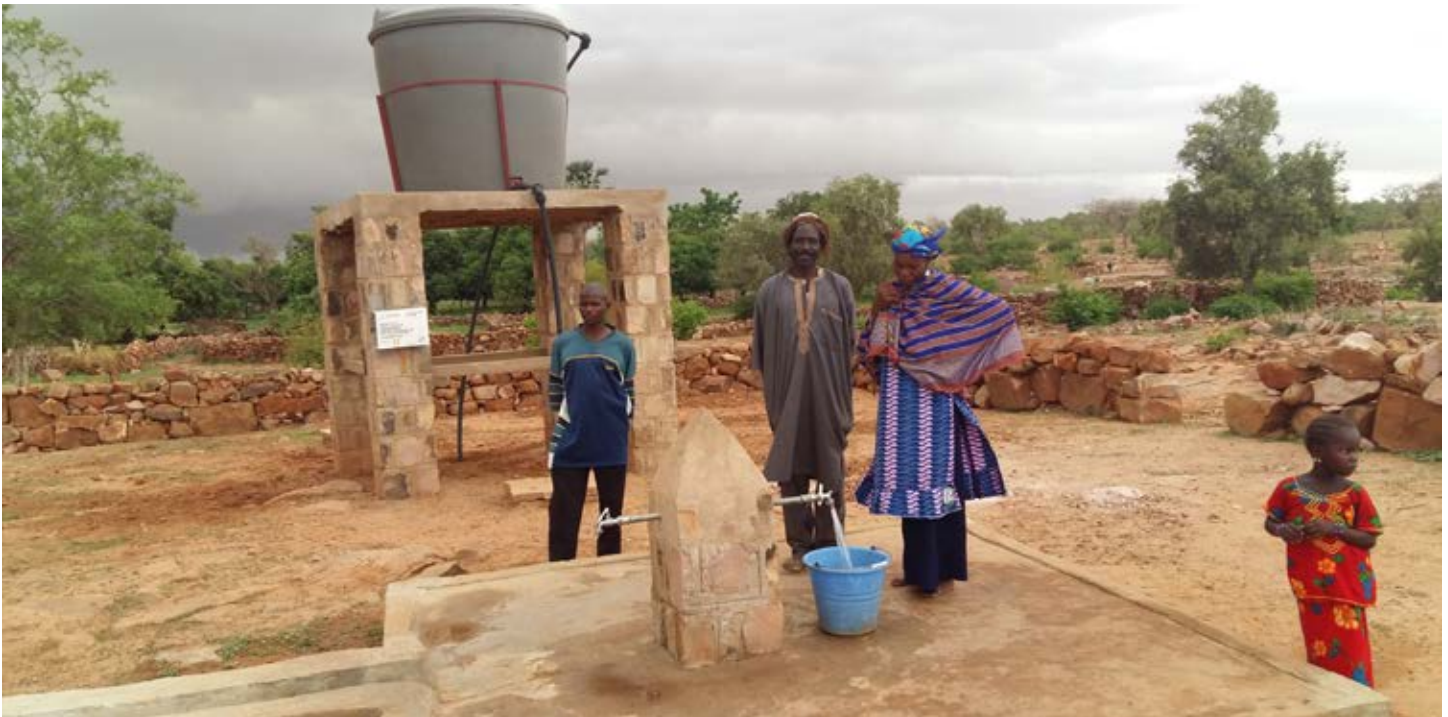
USAID works with local artisans in communities like Anga, Mali, to repair or rehabilitate artesian drilling, such as this one, as an incentive to become open defecation free-certified. Photo credit: CARE Mali
