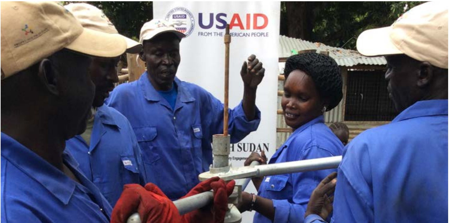
A female pump mechanic helps repair a borehole in Jebel, South Sudan. The borehole was brought to her community through the USAID PROPEL project. Photo credit: USAID PROPEL Project
