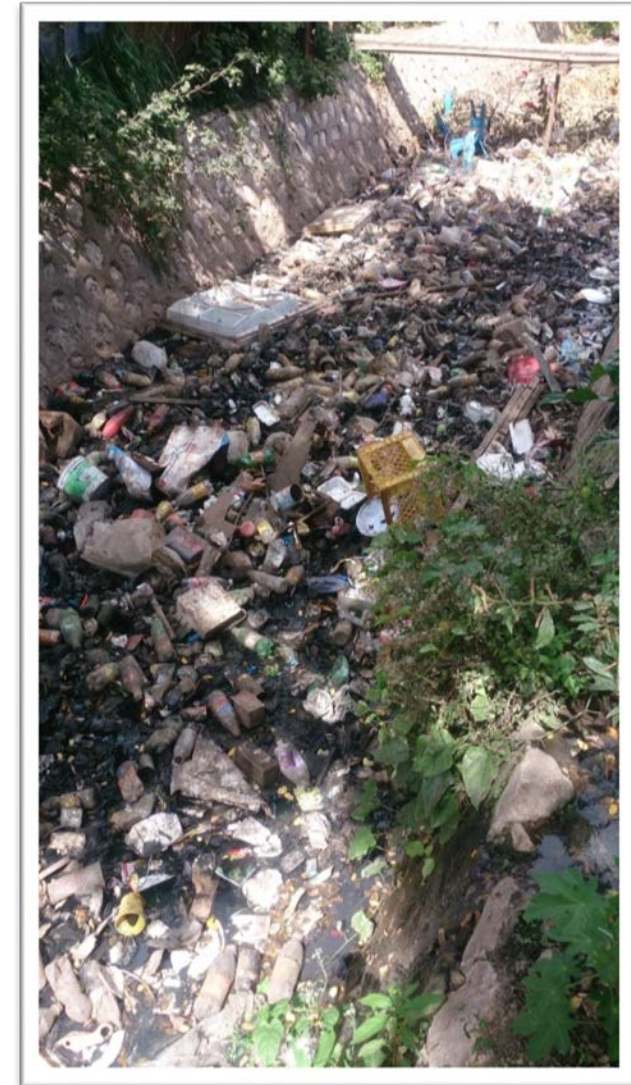
The gully which borders the community
