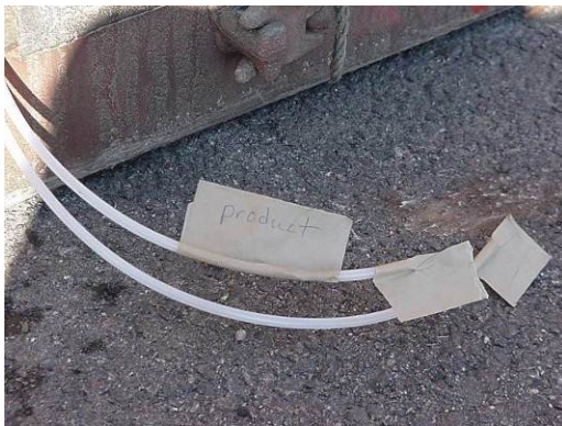
Gas Monitoring Lines
