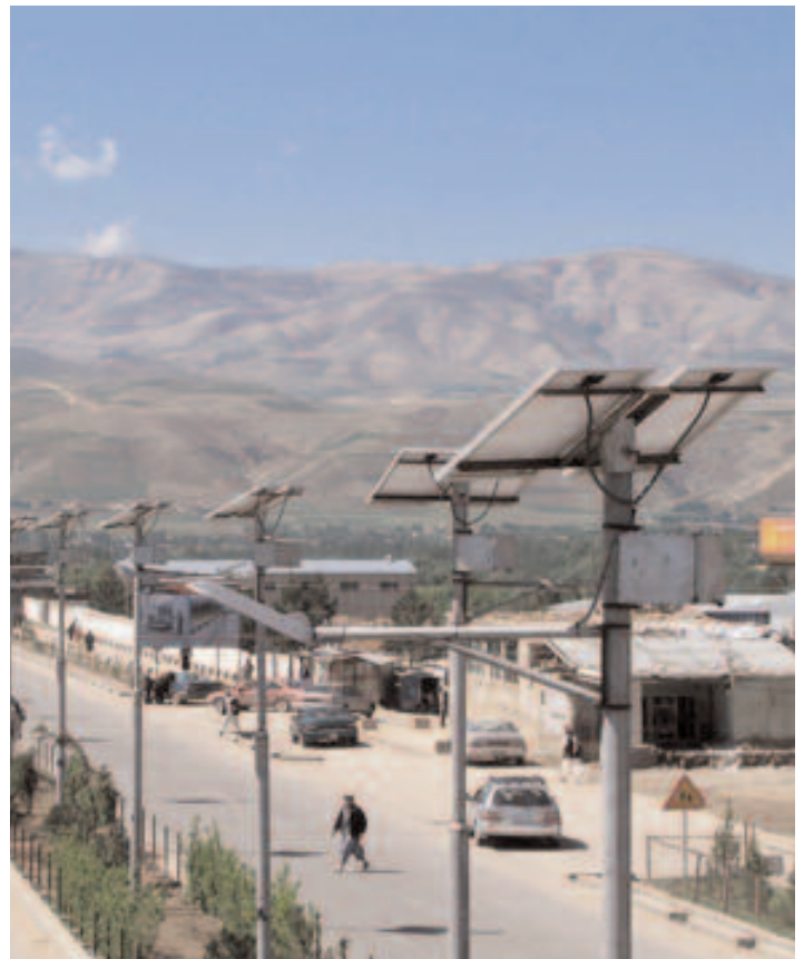
The solar streetlights in the city of Faizabad, located 600 kms from Kabul, were procured and installed under the USAID-funded Afghan Clean Energy Project (ACEP). The city is not connected to the national power grid. Credit: Abdul Raso.
